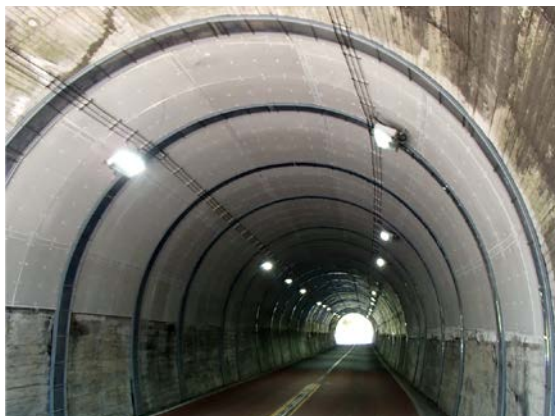
The tunnel is lined with carbon fiber sheet panels to strengthen it (mountain tunnel).
