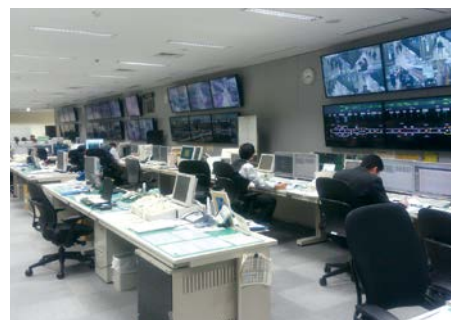
Integrated Control Center
