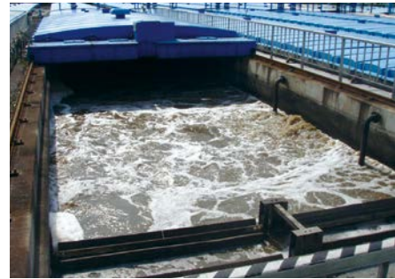
Example of reaction tank
