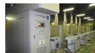
Micro-gas turbine generator
