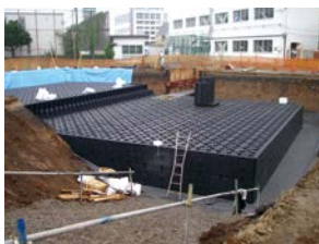
Rainwater storage facility under a schoolyard
